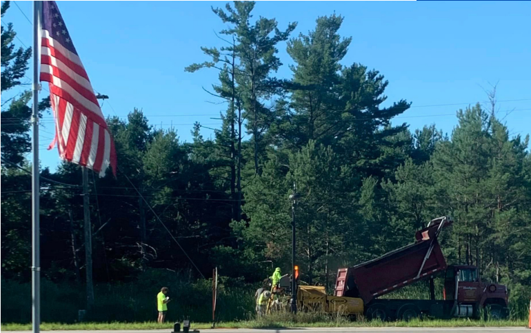
Finished in the Autumn of 2023 the M-55 Pathway was paved and completed/ The pathway leads from the I-75 Business loop / M-55 intersection to the Ogemaw Hills recreation facility
