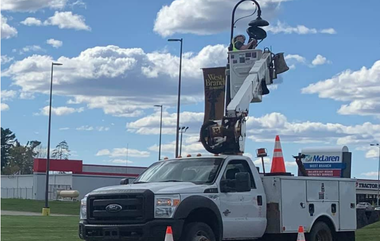
Repairs and Maintaining of the West Branch Township DDA lights continued into 2023 with work by Primary Electric. Repairs continue to included head changes and replacing down poles as needed.
