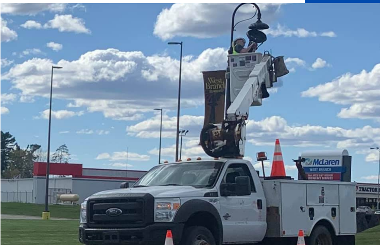
Repairs and Maintaining of the West Branch Township DDA lights continued into 2022 with work by Primary Electric. Repairs included head changes and replacing down poles.
