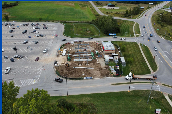
Approved in Early 2022 construction has been moving well this summer on the New Murphy Gas Station located in front of Wal-Mart in the DDA District.
